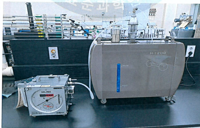
Fig. 1 Equipment configuration installed in KRISS at Hue Light Co., Ltd.
